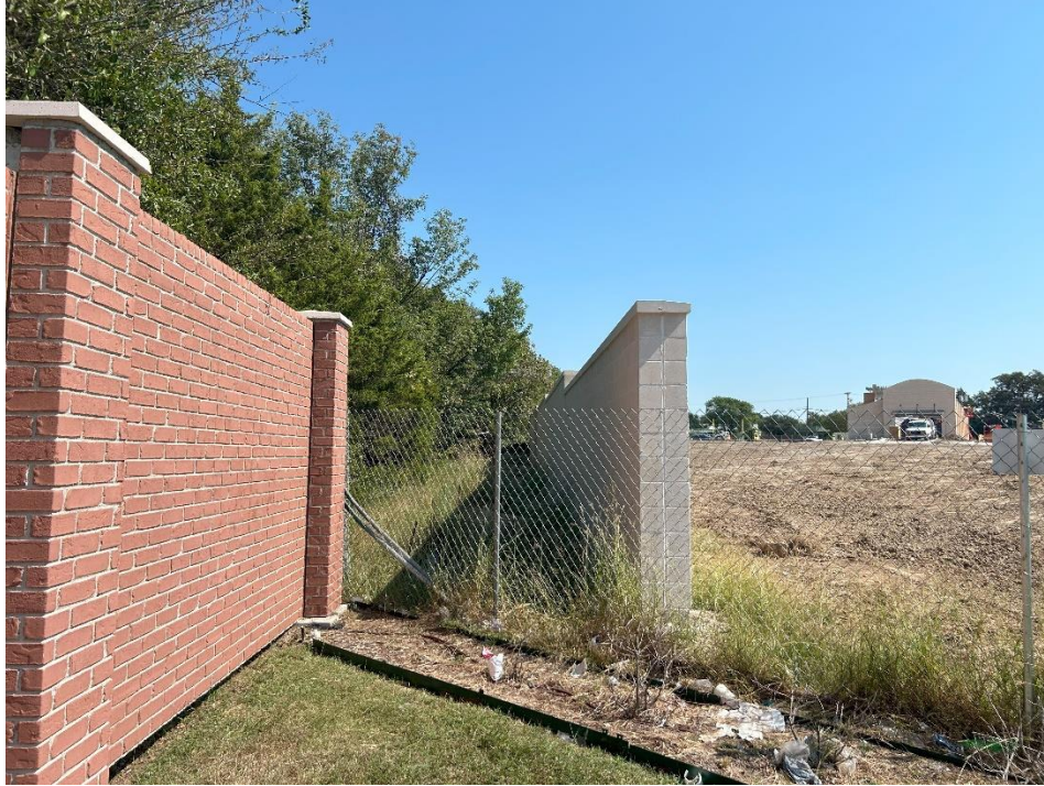
Gap between Golden Chick and Superstar Carwash Wall
